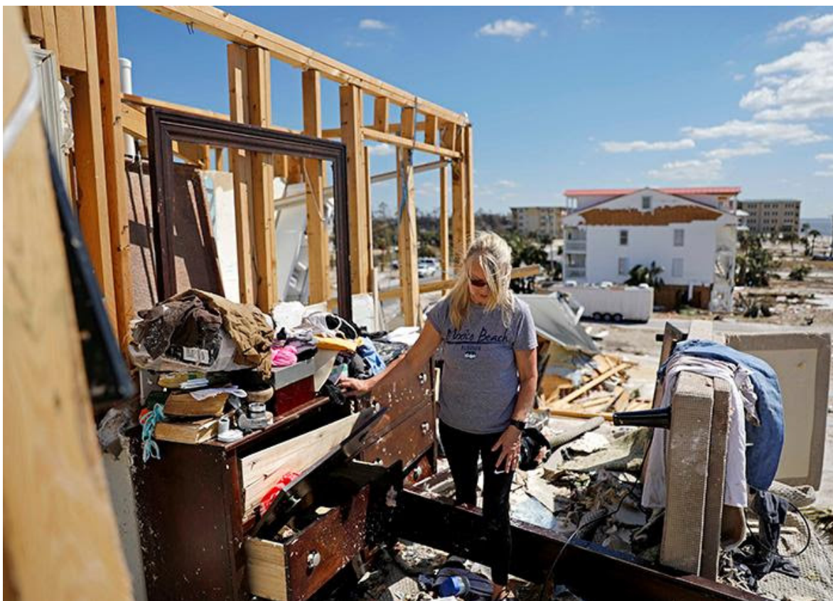
A resident of Mexico Beach, Fla., sifts through what was her third-floor bedroom while surveying damage from Hurricane Michael on Sunday. | David Goldman/AP Photo
