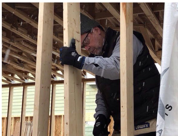
Hammering nails on a snowy day in January 2019 to frame a wall in the duplex we were building for Habitat for Humanity.
